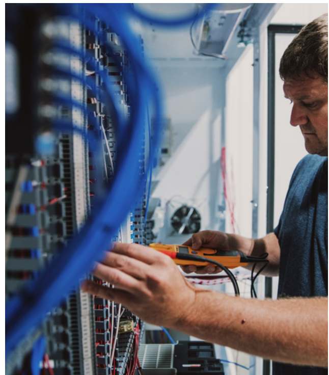
Every Control Panel is built and tested at the Airvac facility. Customers have the option to tailor the control panel to their specific needs.
